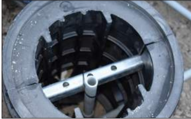
Conduit can be tie wrapped or wire tied to the middle bar for support.
