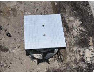
Gravel filled in, in 3"-6" (76 mm - 152 mm) increments, and then hand- or machine-tamped.
